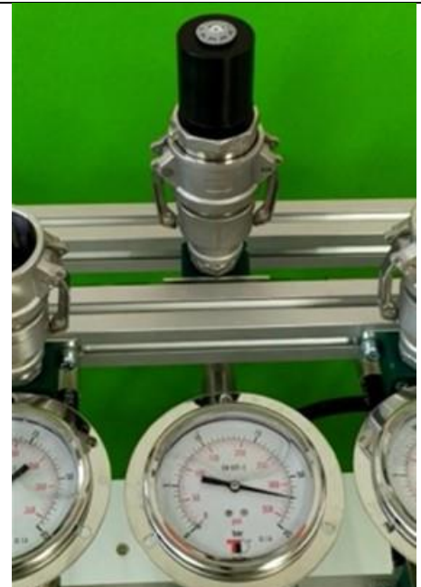
[Figure 3] Complete testing installation
